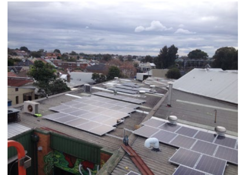
Young Henrys brewery rooftop solar array, Sydney NSW Photo courtesy of Pingala
